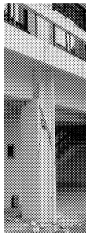
1st-floor support column in 2-story building fractured
